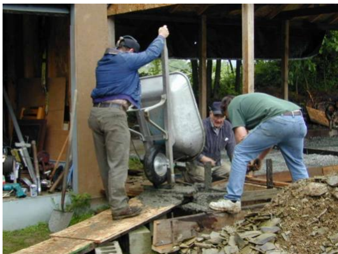
It took a large hole, a lot of wheeled in concrete, and a lot of tamping (N3OS was not a short guy)
